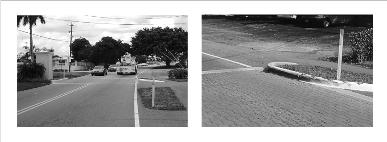
Figure 6.12. Problem Choker Prior to Improvement. (Ft. Lauderdale, FL)
