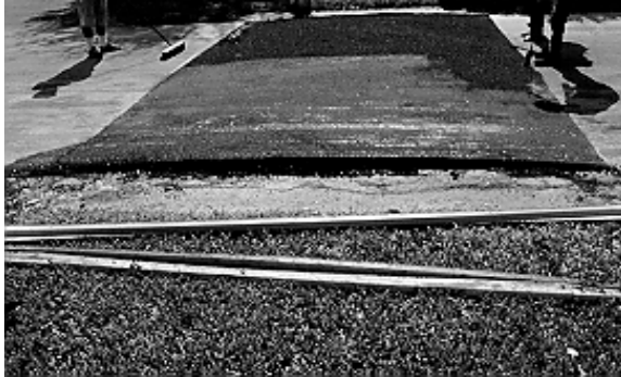
Figure 4.5. Use of Cutout to Replicate the 12-foot Parabolic Hump Profile. (Ft. Lauderdale, FL)
