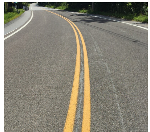
Figure 3. High friction surface treatment at a curve in Foster, RI. Source: RIDOT.
