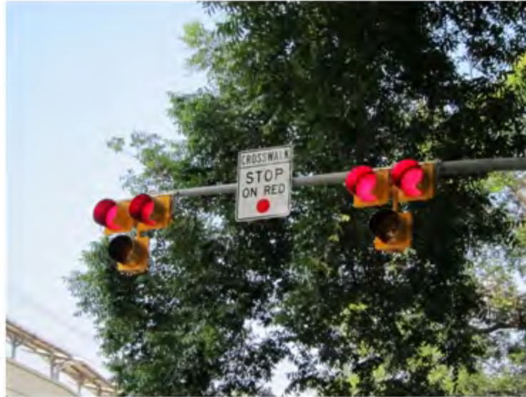
Exhibit 5-13. Pedestrian hybrid beacon. Source: FHWA Office of Safety
